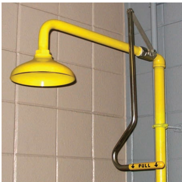
FIGURE 5-10 Safety shower for removing toxic chemicals. Source: Delmar/Cengage Learning.
